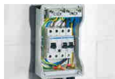
British Standard installation with earthed armoured cables
