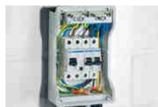
British Standard installation with earthed armoured cables
